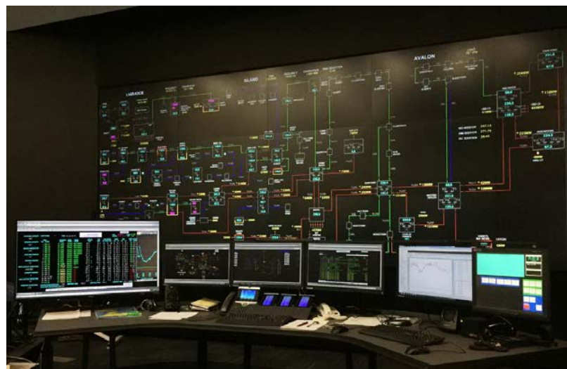
Figure 4: ECC One Line Display (Post Upgrade)
