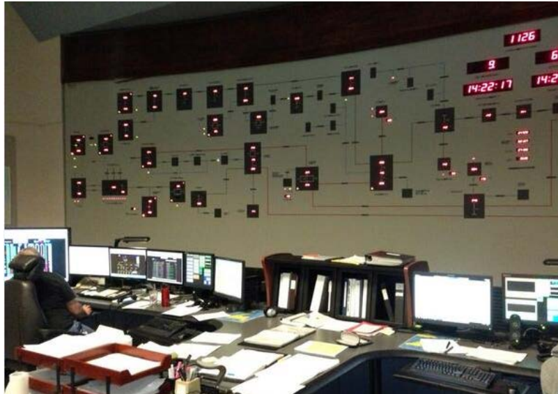
Figure 3: ECC Display (Pre Upgrades)
